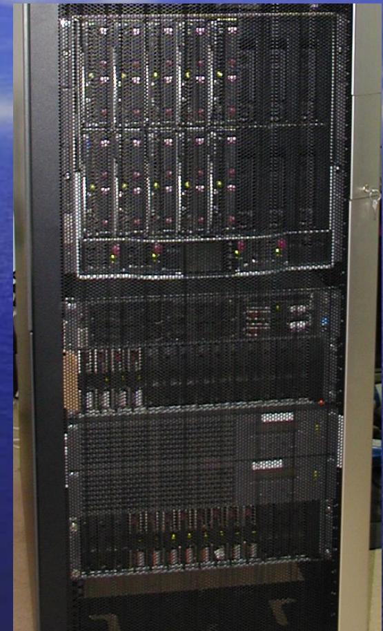
Xeon-based blade servers with SAN/NAS storage
