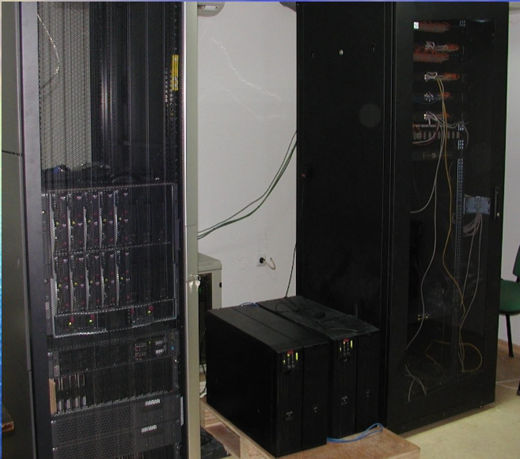
A view of the basic server/LAN infrastructure area
